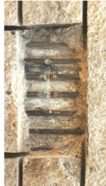
Sonic/ultrasonic measurements effective in detecting cut pre-stressing wires; subsequent tests indicate that the mortar coating and adjacent uncut wires kept the pre-stress in tension away from the cut areas. Image courtesy of Lewis Engineering and Consulting, Inc.
