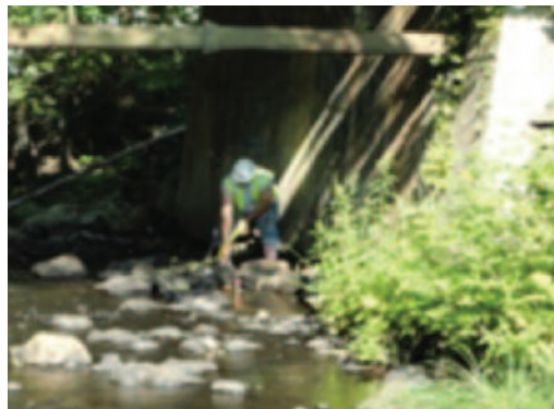
NDT crew conducting seismic refraction testing to profile bedrock at the abutments of a bridge with an unknown foundation.
