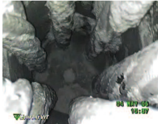
Void PT duct at Anchorage.
