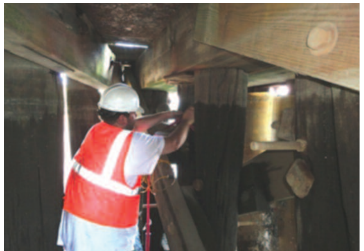
NDT technician attaching sensors to a timber pile for pulse echo measurements to determine pile length and length of embedment.
