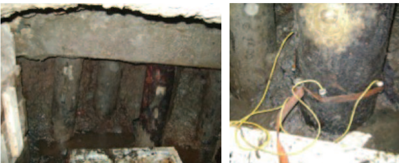
NDT Corporation determines how deep a pile foundation is. Typically these measurements are made in conjunction with a geotechnical test pitting and boring program.
