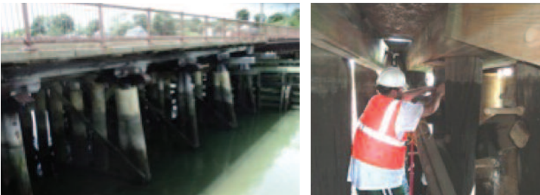
NDT Corporation using pulse echo measurements on timber and sheet piles to determine their lengths.
