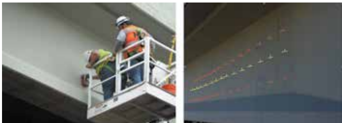
Fig. 2—(a) GPR to locate web tendons; and (b) tendon locations marked on girder web.
