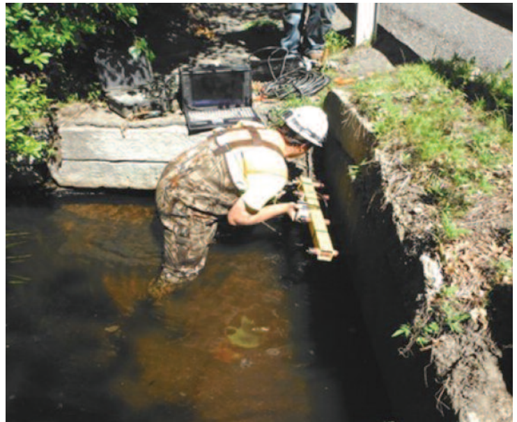
Sonic/ultrasonic pulse velocity measurements being taken on a bridge in the field.
